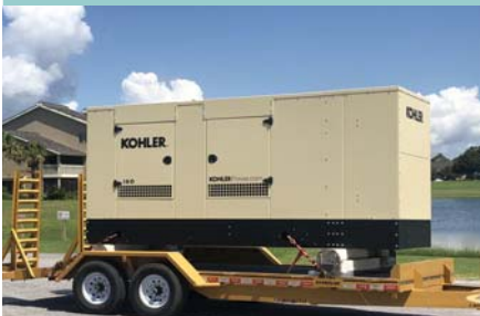
Photo above: Lift Station generator
