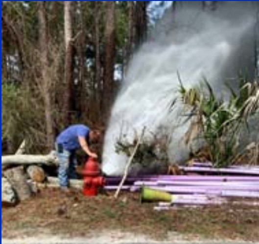
Fire hydrant flushing operation
